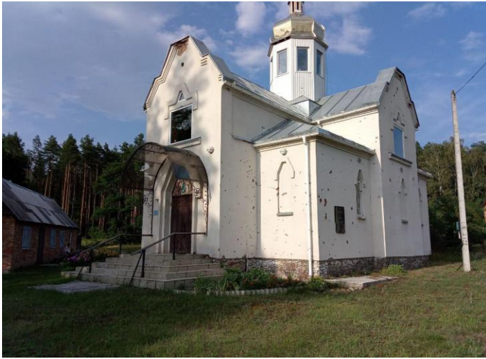
Shrapnel-damaged Church of John the Baptist, Moshchun (Kyiv region). Photo by Kateryna Zorya, August 11, 2022.
