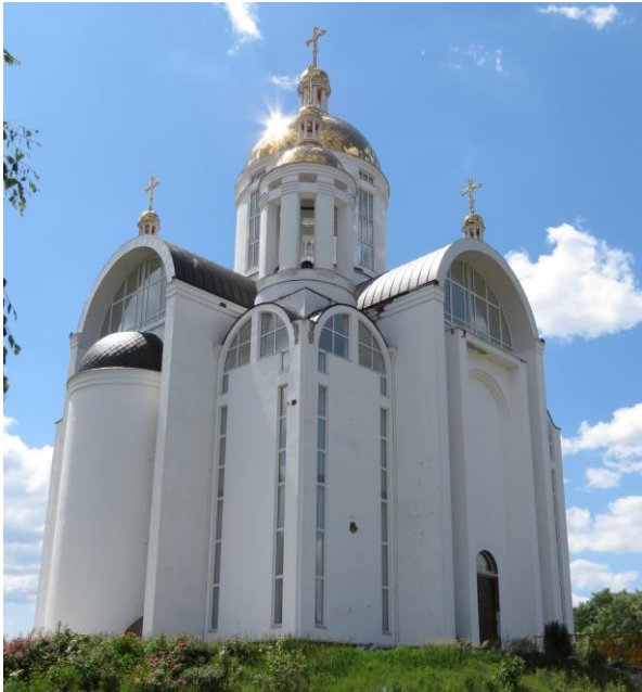
Damaged walls by large shrapnel at the Church of St. Andrew the Apostle the First-Called and of All the Saints, Bucha (Kyiv region). Photo by Ruslan Khalikov, June 25, 2022.
