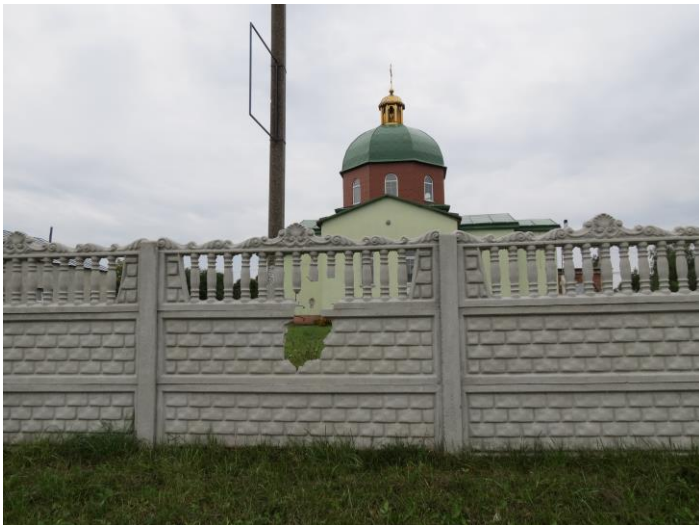
Church of St. Nicholas the Wonderworker Church, large shrapnel damage, Nalyvaykivka (Kyiv region). Photo by Ruslan Khalikov, September 17, 2022.
